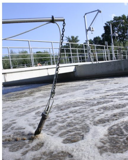
An IQ SensorNet dissolved oxygen sensor deployed directly in the aeration basin for continuous monitoring and control of aeration.
